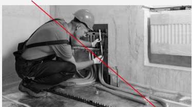
Laying pipelines Wasting Time, Labor, Money
